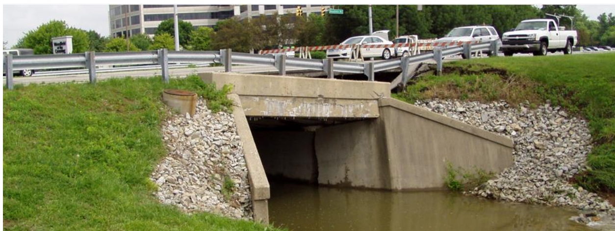
Figure 152. Fluvial Erosion Example (from http://feh.iupui.edu/ )
