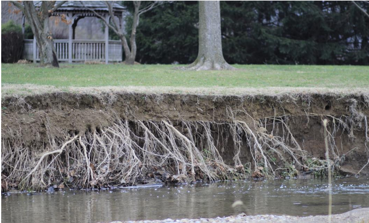
Figure 153. Fluvial Erosion Example (from http://feh.iupui.edu/ )
